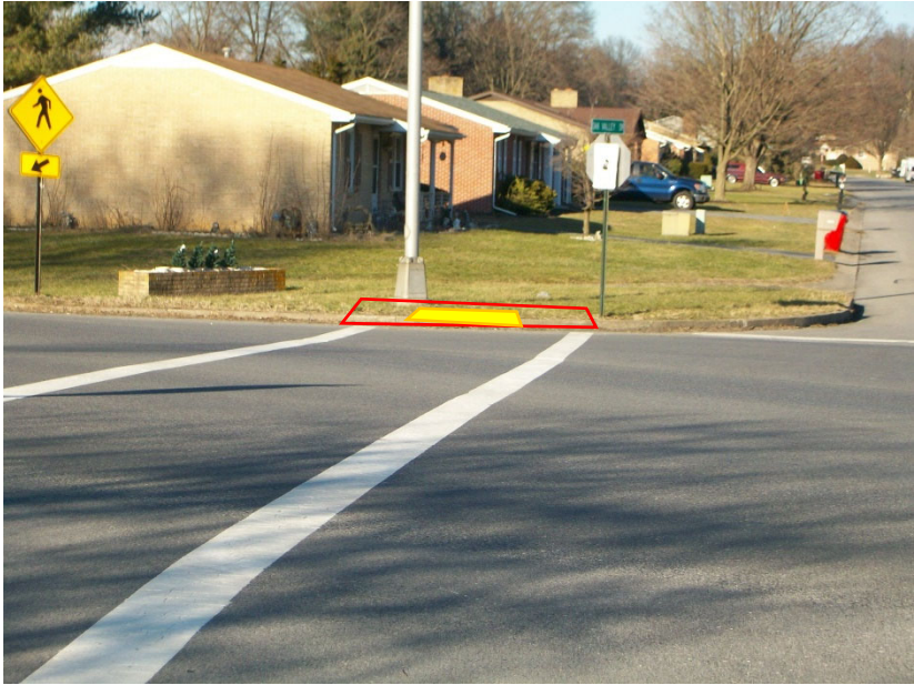
Halfway Boulevard at Marty Snook Park: Construct Parallel Ramp STD. No. MD 655.12
