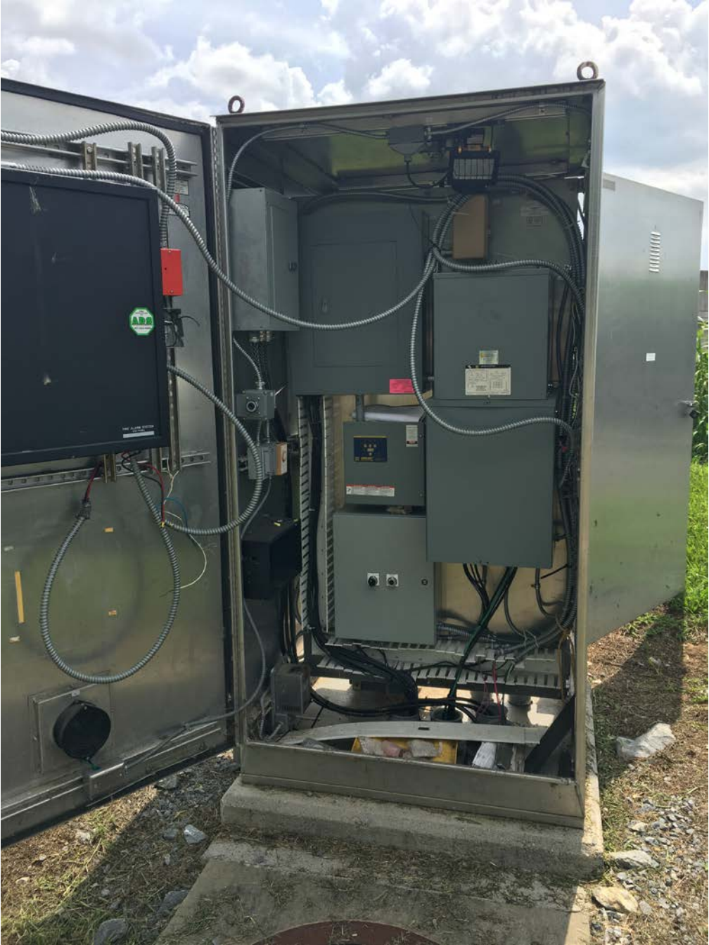
Photo 4: Other side of Electrical Cabinet
